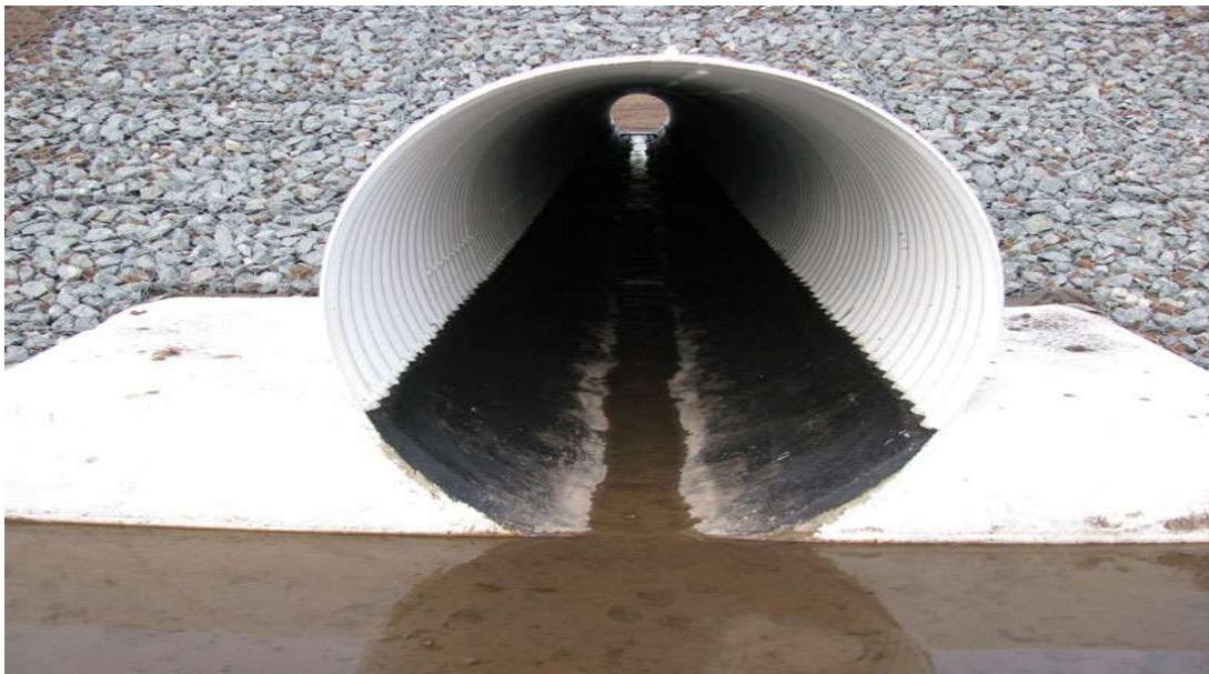
Figure 3 Corrugated water pipe.
